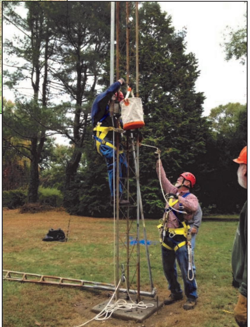
KB1JEY completes the work on the top of the lower section prior to it being lowered.
