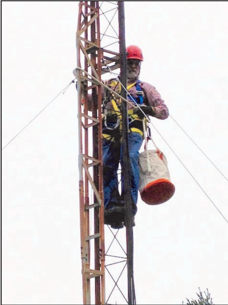
K3TUF led the crew through the take-down. Here at the hinge he lubricated the hinge bolts to ready it for tilt over and antenna and upper section removal.
