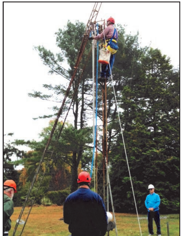
K3TUF directing upper section lowering — the most critical point. Once the gin pole was attached, the lever arm was separated from the upper section and lowered to the ground. Then the hinge bolts could be driven out and the upper section carefully lowered. Lowering in stages kept the operation (relatively) safe.
